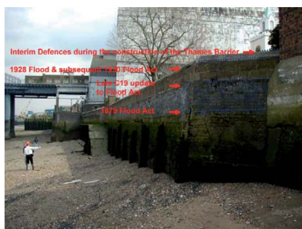
Figure 20: A traditional response to floods can lead to progressive unplanned adaptations, as seen here in the Thames a series of flood events lead to the need to raise and re-raise the flood walls
