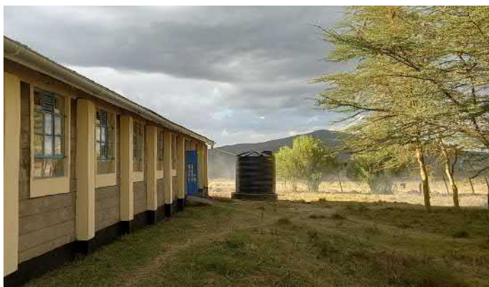
Rainwater Harvesting system installed in Nkineji Primary School, Siana
